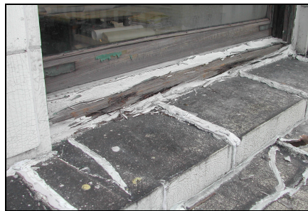
Cracked terra cotta windowsill.
