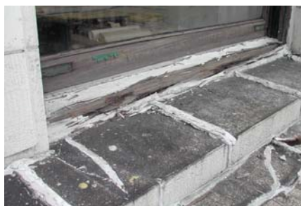
Cracked terra cotta windowsill.
